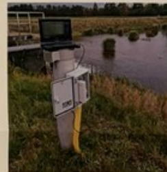
Figure 3: Soil Moisture sensor towards the inlet
